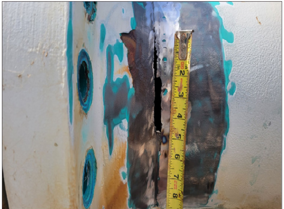
Figure 4: Leaking Raw Water Pipe Requiring Repair During 2022 Drawdown at the West Hackberry Strategic Petroleum Reserve Site
