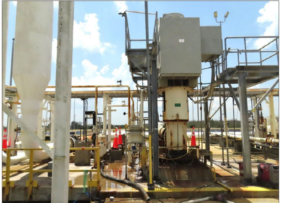
Figure 7: Leaking Brine Disposal Pumps at the Big Hill Strategic Petroleum Reserve Site
