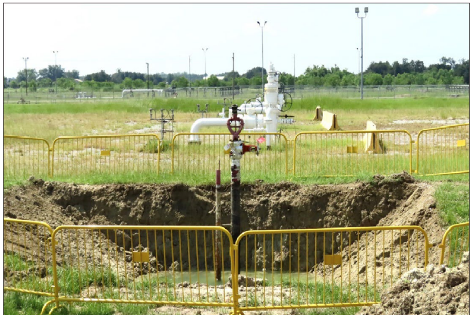
Figure 6: Leaking Fire Suppression System at the West Hackberry Strategic Petroleum Reserve Site
