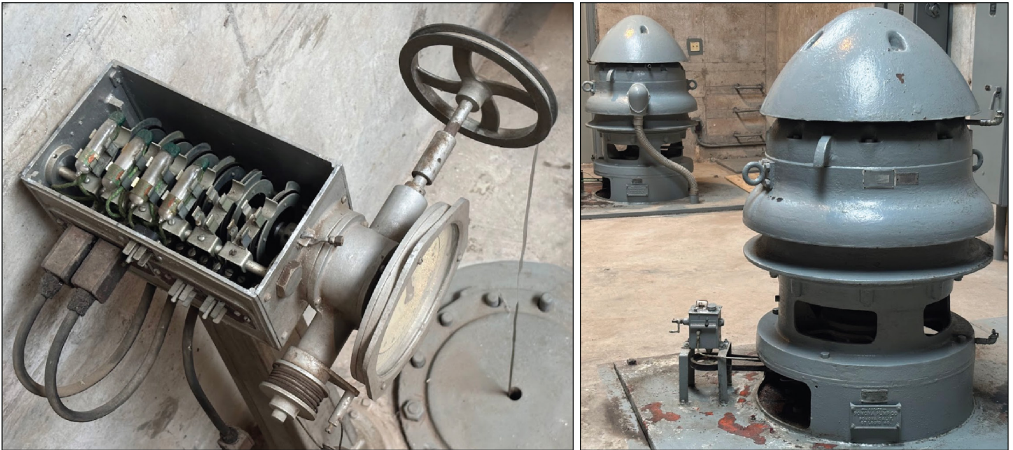
Figure 15: Approximately 80-Year-Old Pump Station Equipment to Be Modernized in Tulsa, Oklahoma
