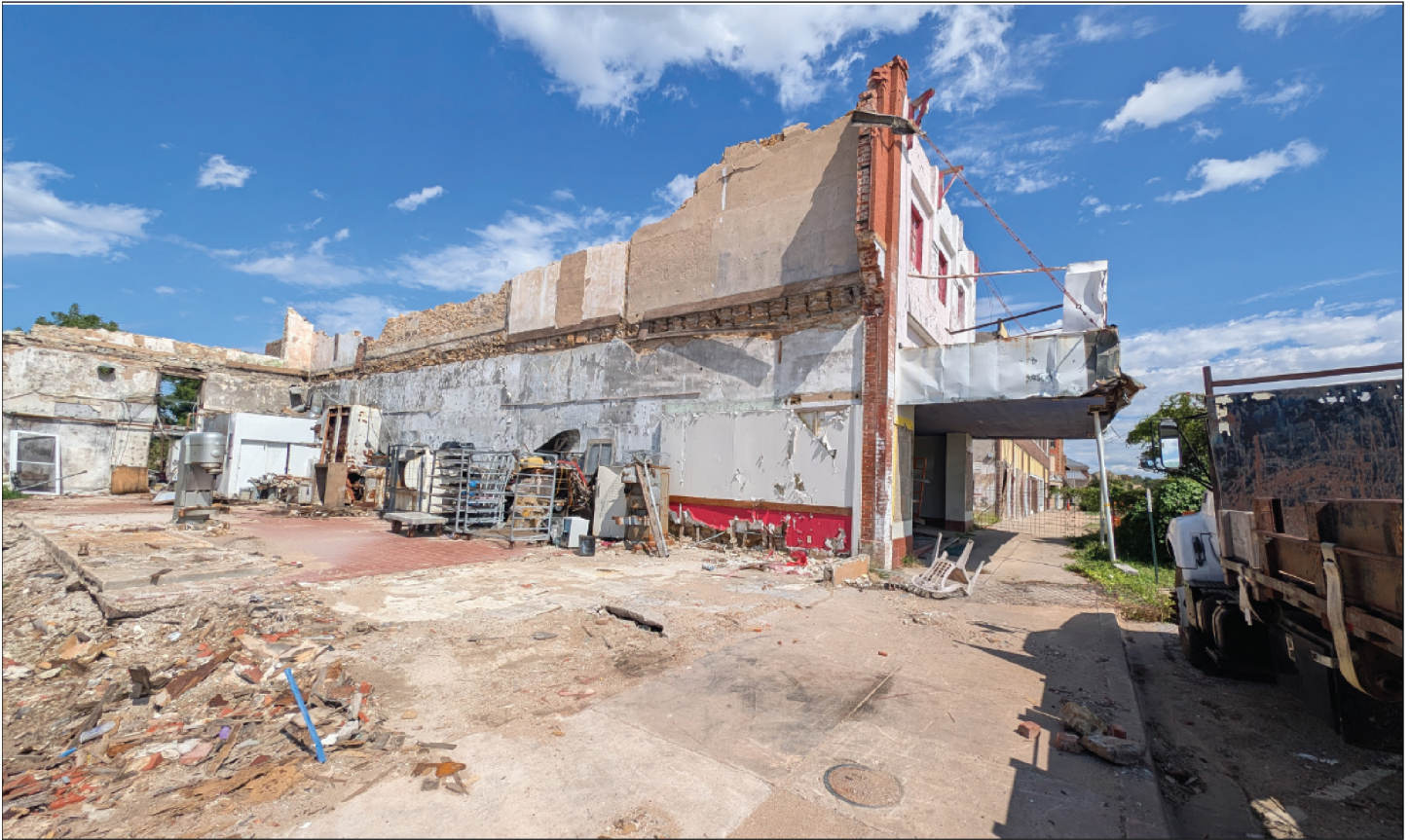
Figure 3: Damaged Business in Downtown Sulphur, Oklahoma, About 1 Year After 2024 Oklahoma Tornadoes
