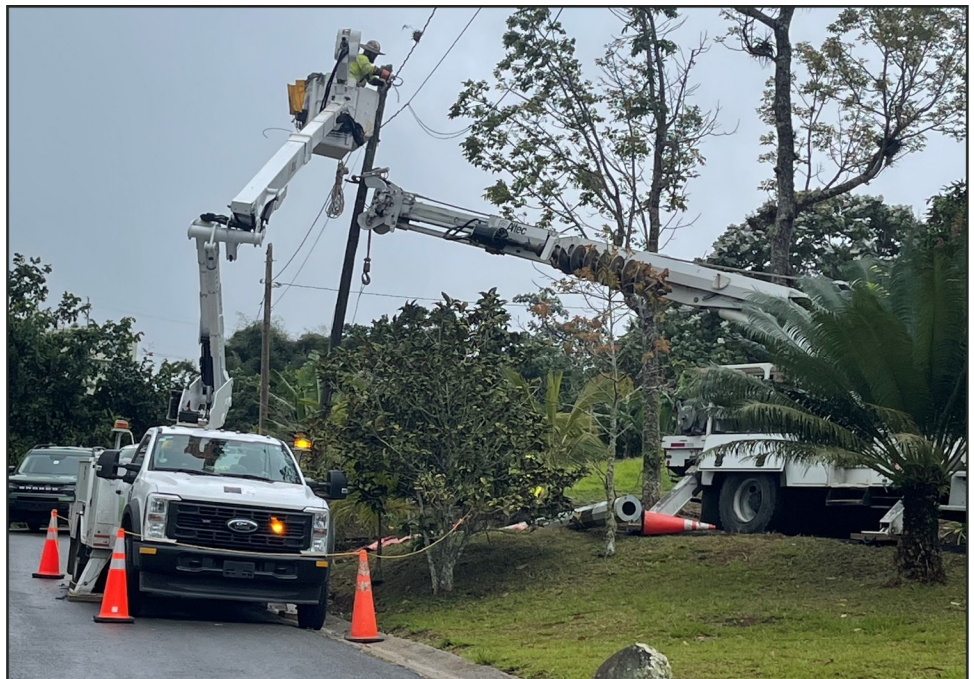
Figure 2: FEMA-funded Pole Replacement and Streetlight Repair Project in Coamo, Puerto Rico (February 2025)
