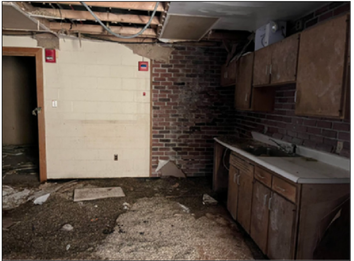
A derelict building at the Long Range Navigation (LORAN) station in Caribou, ME.
