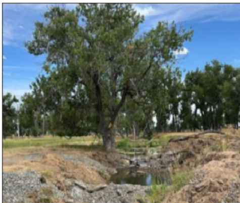
Engineered stream to improve aquatic habitats and access to water by bison, and reduce erosion as part of the Bison Management project in Colorado.
