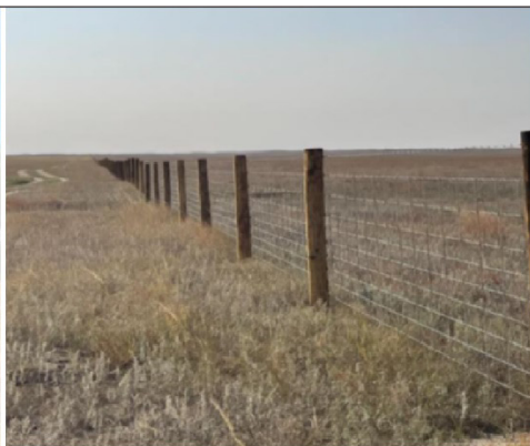
Construction of fencing to improve bison management as part of the Bison Management project in Nebraska.
