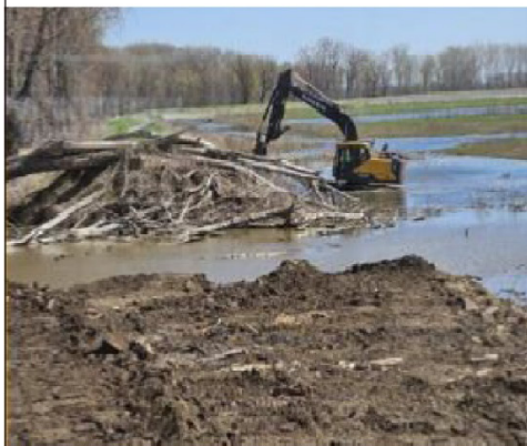
Repairs to levees and spillways, structures to provide for the controlled release of water, to reduce risks from flooding along the Mississippi River in Illinois as part of the Upper Mississippi project.
