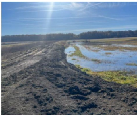
Work on and around a levee in Tennessee, including regrading low areas to improve drainage, to better manage ponds and wetlands used by wintering waterfowl as part of the Lower Mississippi project.
