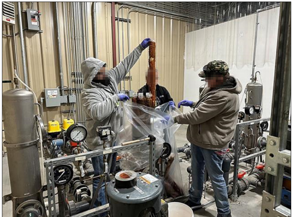
Figure 9: Pump-and-Treat Facility at Hanford Site for Groundwater Cleanup
